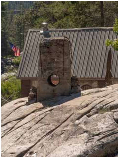
Top picture: more concrete supports for the pipe from the reservoir/pond to the generator building. Middle: a view of the dam late in the season. Bottom: the last concrete support with the generator building in the background.
